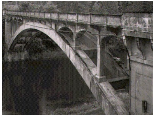
Baker River Bridge (WA-105). State Route 20 spanning the Baker River - City of Concrete, Skagit County Built, 1917. Unknown Photographer, Courtesy of Washington State Department of Transportation (WSDOT).
