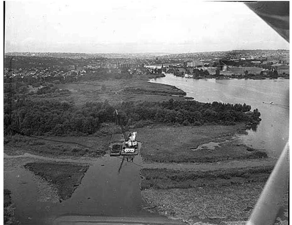
Dredging the site of the west approach bridge structure (1961) Photo courtesy of MOHAI, Seattle P-I Collection, image no., image no. 1986.5.7575.2
